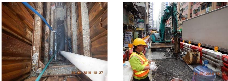
Cheng and his team had to excavate the road surface to replace the defective sewer located six metres underground.
