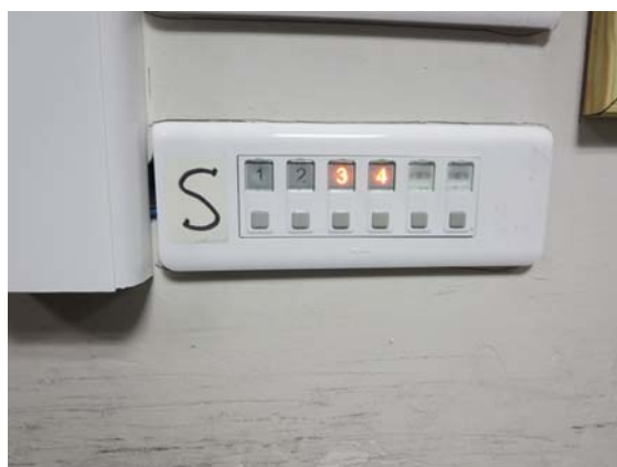
Call control board at Ilundáin, Aranguren (Navarre)
