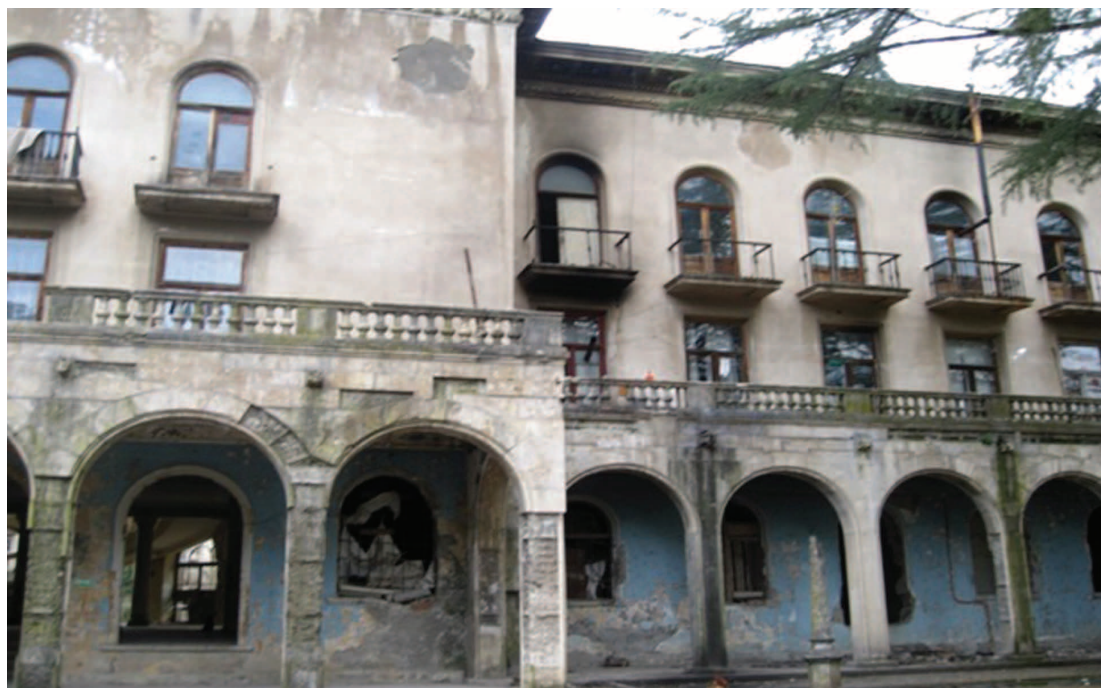
Tskaltubo “Sanatorium Imereti”. The building is wrecked. Transfer of IDPs had not occurred.
